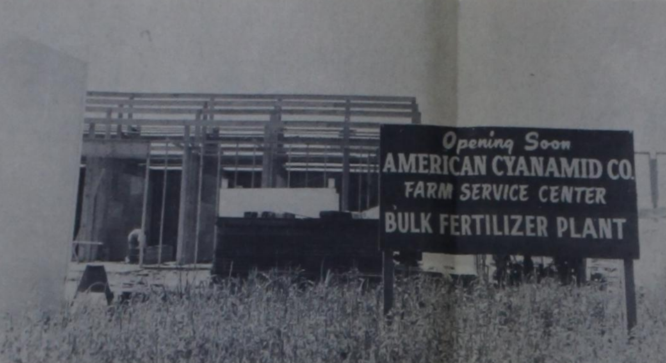
NOW GOING UP on US 385 in North Dimmitt is an American Cyanamid farm service outlet and fertilizer blending plant. Constructed by Brown & McKee Construction Co. of Lubbock, the 50 by 120 ft.
