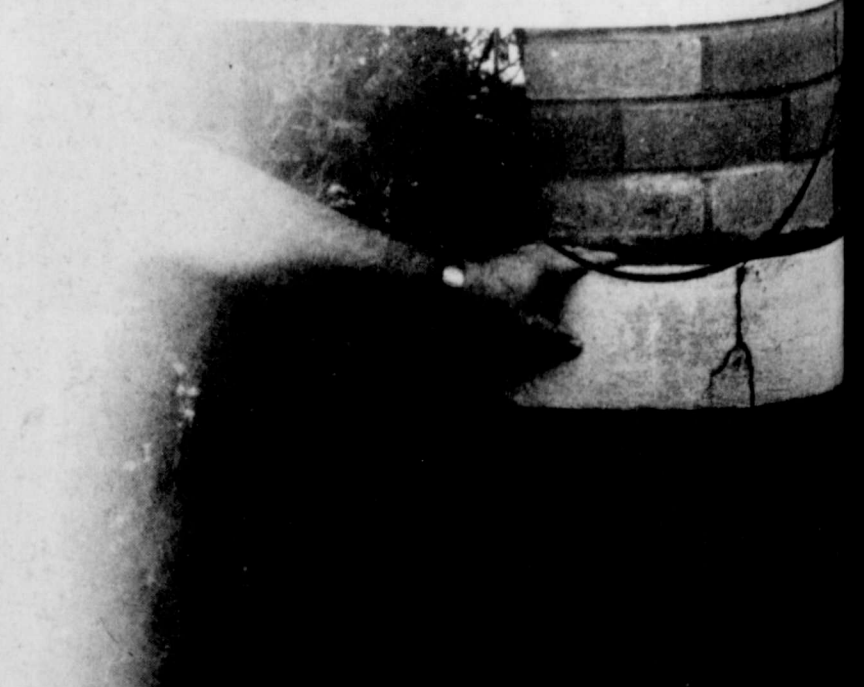
DEPUTY SHERIFF SHOWS large crack in n.w. corner of jail foundation settling.
