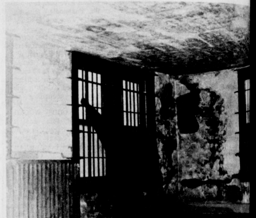
N.E. CORNER OF 3rd FLOOR cell block, missing plaster & ceiling due to rain seeping in through cracks in exterior walls, moisture from open showers located on the same floor.
