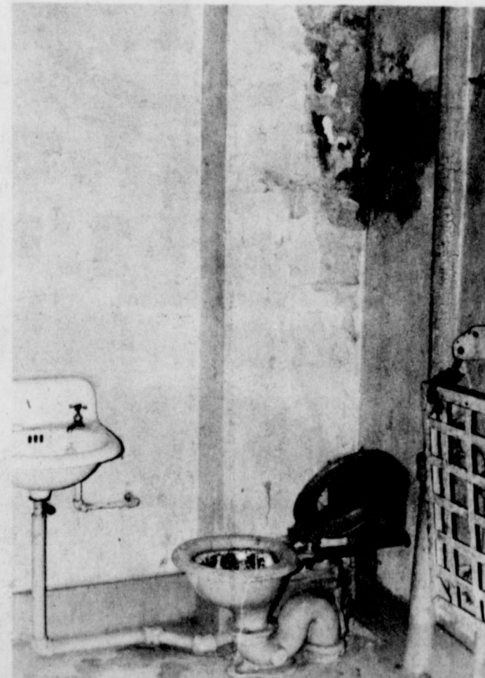
SECOND FLOOR CELL shows more wall deterioration due to moisture.
