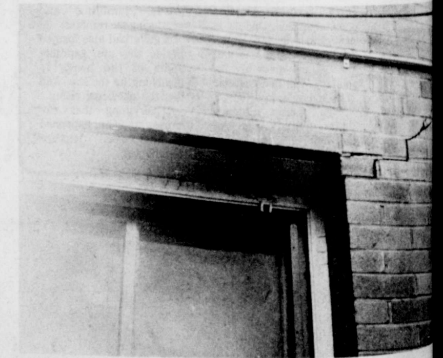
EXCESSIVE CRACKING around windows & various corners of cell block due to rain to be blown in behind plaster & mortar type walls, and deterioration of interior walls.
