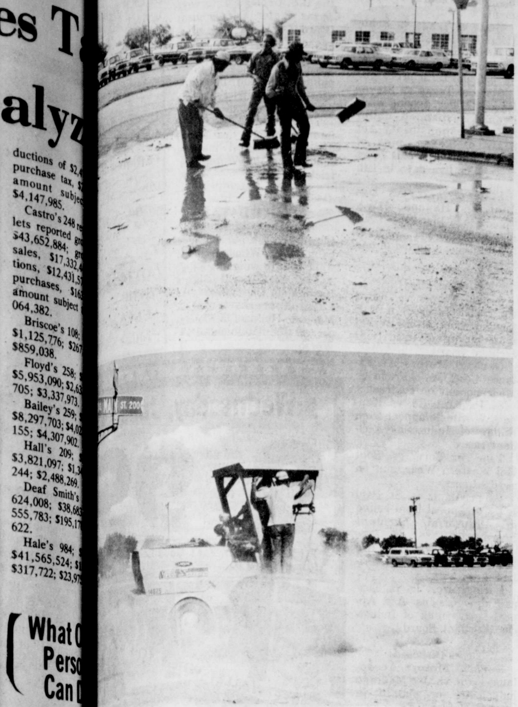
STILL WET from recent rains Thursday morning when workers sweeping Main Street ready for a seal-coat job (top photo)...but by that time the sweeper raised a cloud of dust (bottom) as it passed the same way (Main and Bryant). (Staff Photos)
