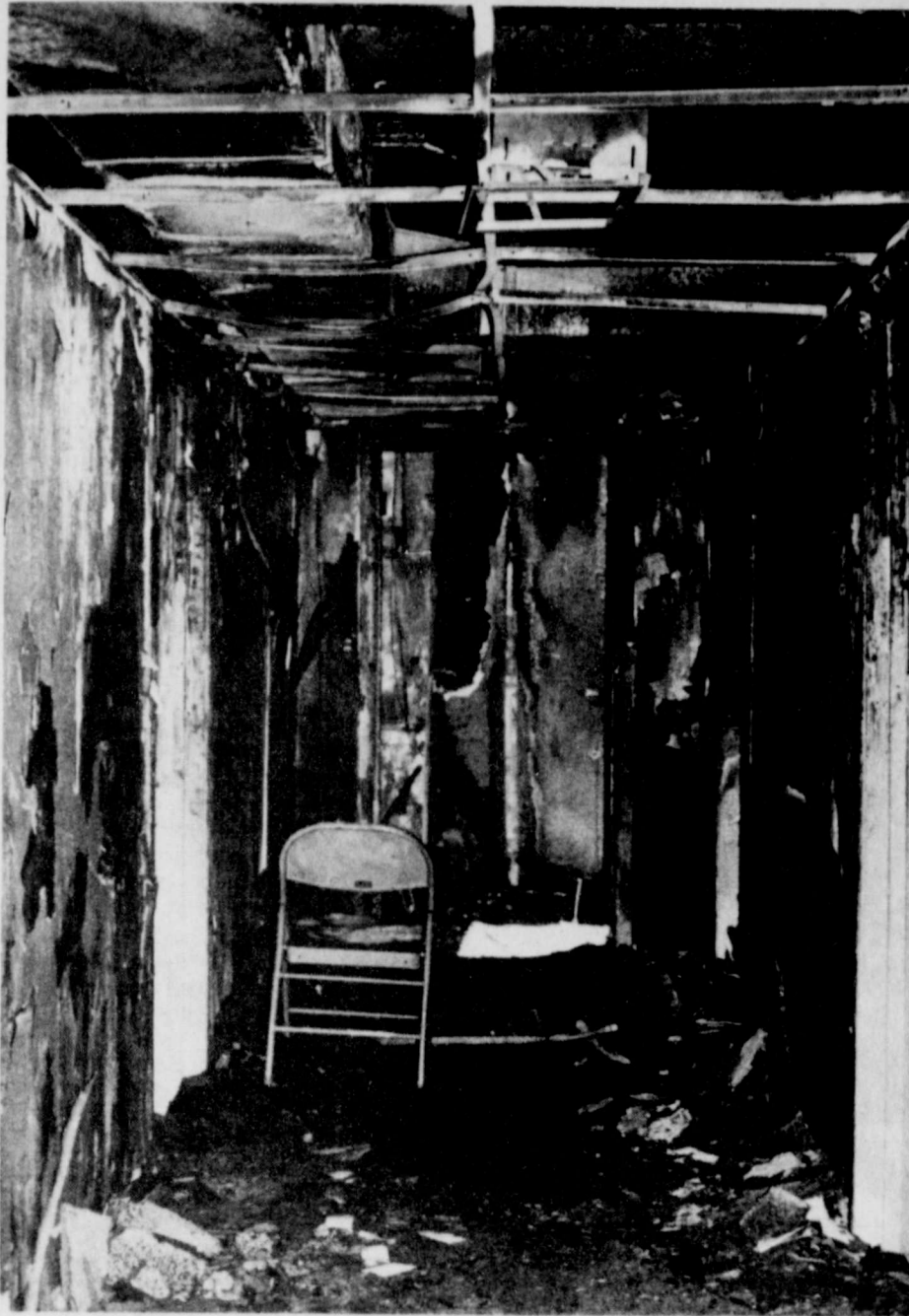
CHARRED HALLWAY at the Aiken First Baptist Church result of Wednesday-afternoon fire. (Staff Photo)
