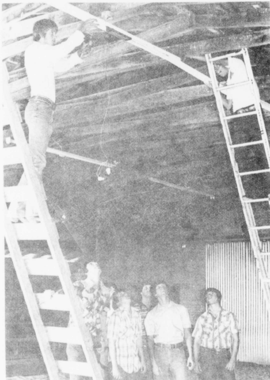
BETTER LIGHTING. . . is in store for spectators and exhibitors at the livestock barn at the fairgrounds this year. Lockney High School VA III class installed new fluorescent fixtures this week. Aaron Wilson and Tim Cooper are on the ladders. "Advisors" are Mitch McMahan, Hector Araujo, Bob Smith, Buddy Wiley, Jody Foster and LaWayne Strickland. (Staff Photo)
