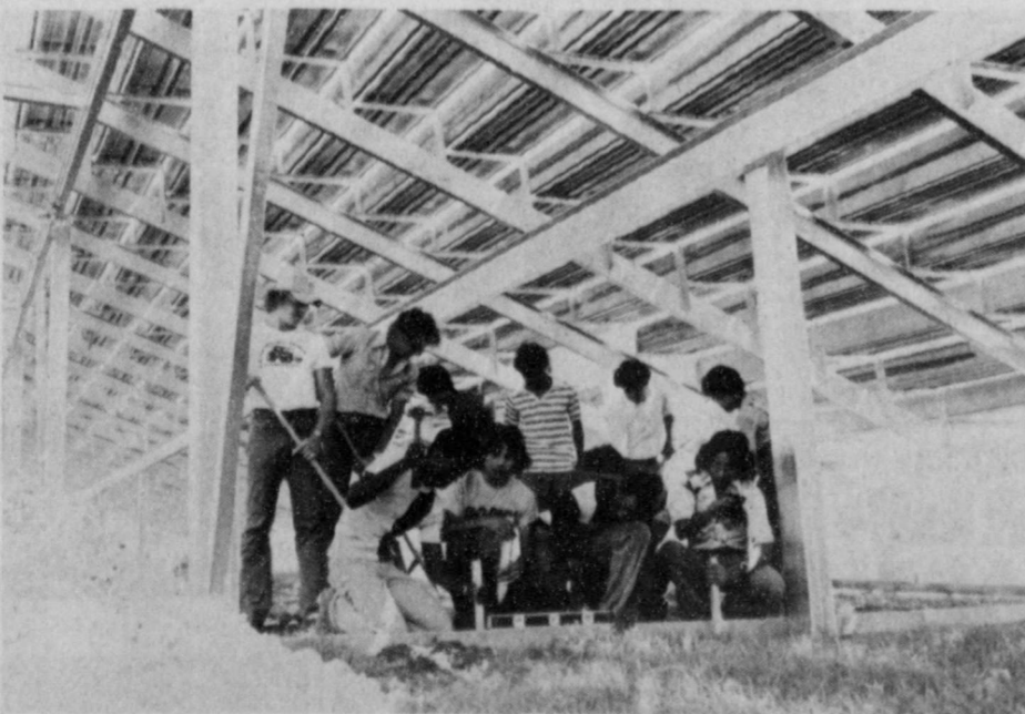
LHS GENERAL AG MECHANICS CLASS was at work last week putting the finishing touches on the stadium-remodeling job. Pictured are (front) Smokey Hill, Robert Gutierrez, Danny Clark, Jessie Nuncio, Jerry Rodriguez; (back) Terry Roberts, Lyndall Stapp, Danny Wilson, Oscar Garza, Joe Rodriguez, Pete Molina. Another class member, Monty Hulcy, is not pictured. (Staff Photo)
