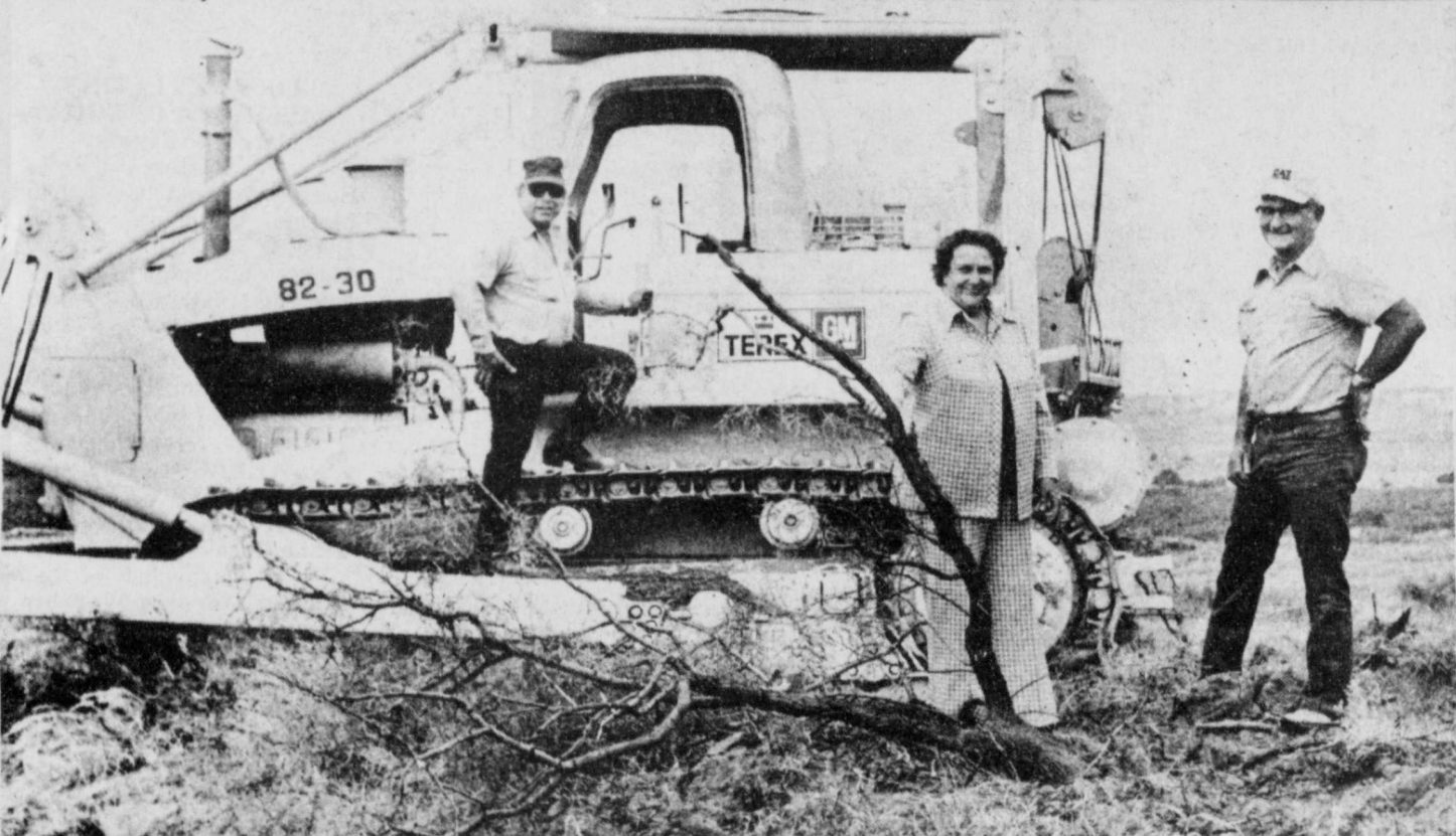
THE INDIANS once rode across this Blanco Canyon plateau, which is being cleared in preparation for the erection of Crosby County's first solar heated and
