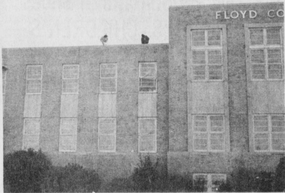
RESTORATION OF THE COURTHOUSE AND AGRICULTURAL BUILDING began this week as Karr Tuck Pointing of Iowa employees place a protective covering over all the windows.
