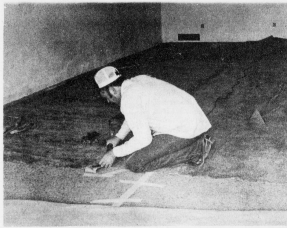
JOHN REDDING has performed the carpet installation at the new establishment for Lovell-Collins this week.
