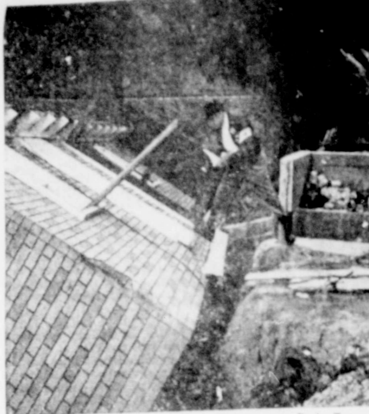
J. H. Green Jr., Red Cross disaster worker from Paris, Tex., inspects the home of R. P. Boyd near Prestonburg, Ky. The home was one of more than 15,000 destroyed or damaged in floods which ravaged Eastern Kentucky, Virginia and West Virginia last January, where Green was assigned to help provide Red Cross assistance to the flood victims. Flood waters of the Leticia Fork of the Big Sandy washed the ground from under the foundations of the Boyd house and destroyed its contents. The Red Cross will rebuild the house and provide household furnishings. As always this assistance is provided as a free gift of the American people, to help the family recover from disaster-stricken areas.
