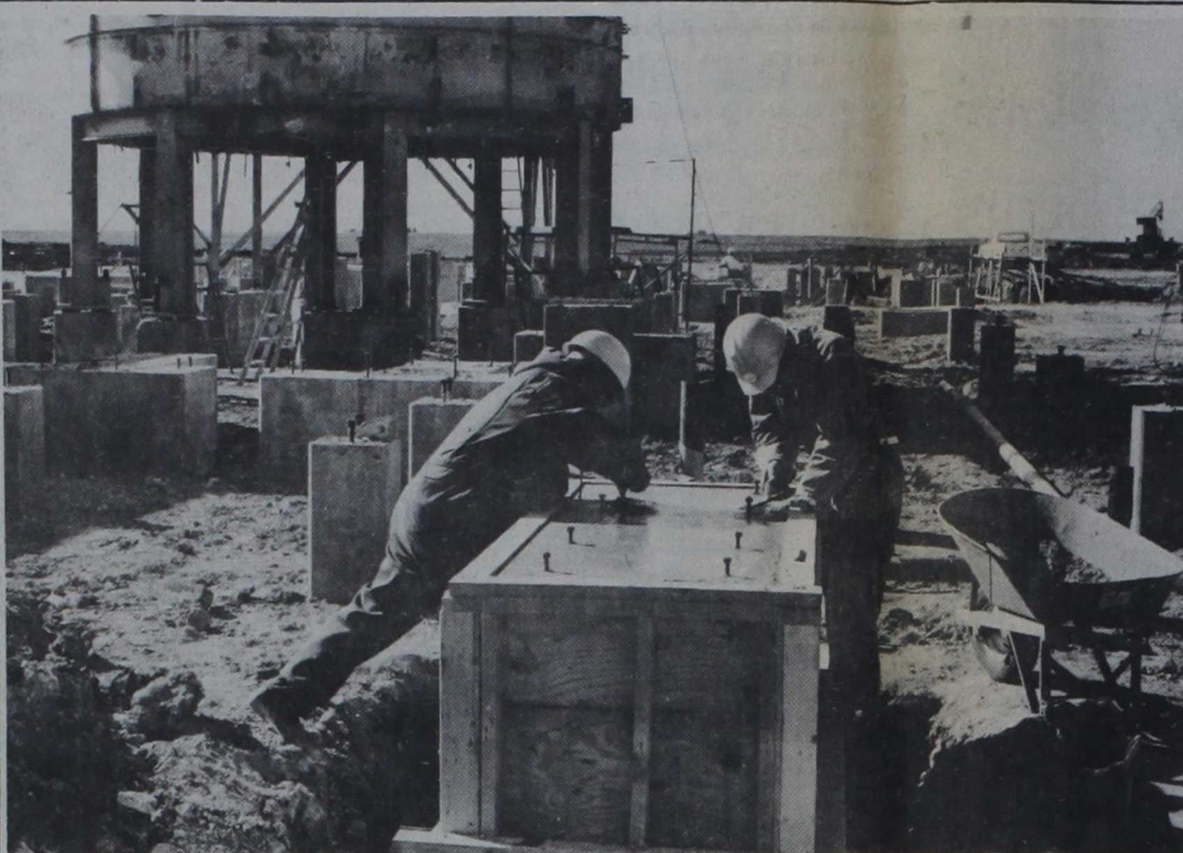
A MONUMENT GARDEN OF concrete pilings is growing at the site of Western Ammonia's new plant expansion. These footings will support the main part of the new plant after a
