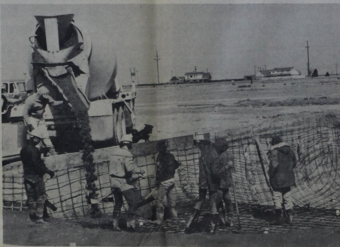
Concrete for every need—Killingsworth Builders Supply pouring concrete for the swimming pool at the Townhouse Addition in southwest Dimmitt . . .
