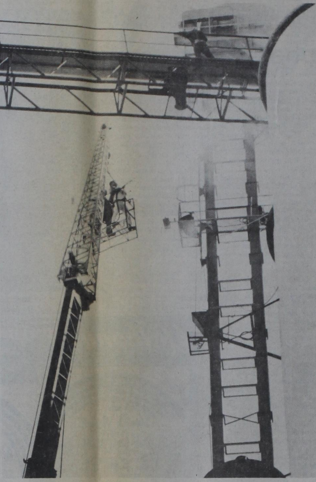
FIGHTING A FIRE while suspended from a crane boom may not be a favorite pastime, but that's what these Dimmitt firemen had to do last Thursday morning when a belt caught fire near the top of an elevator leg at Dimmitt Agri Industries' South Elevator. Welders were working near the top of the leg when the belt caught fire. No one was injured, and damage was held to a minimum.
