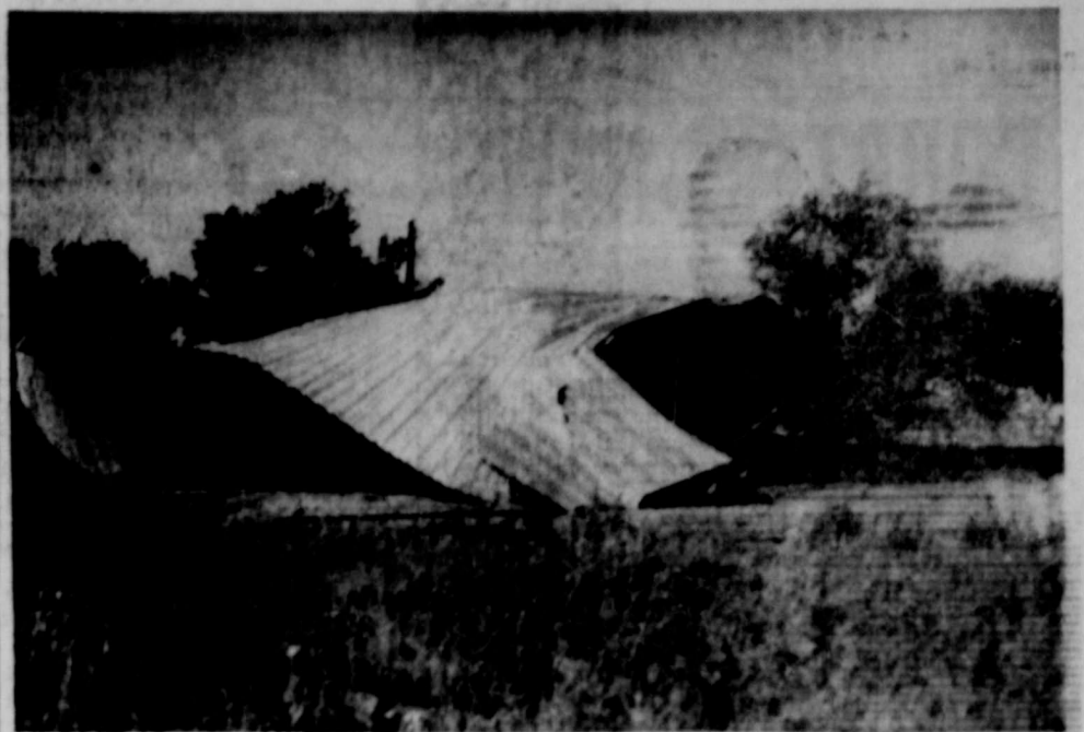
CRUMPLED — The Thompson Pipe Line Co. warehouse in Cisco was blown approximately 100 yards into the Truck Harbor Cafe by high winds Monday morning. The view is looking west. — Photo courtesy of Cotton's Studio.
