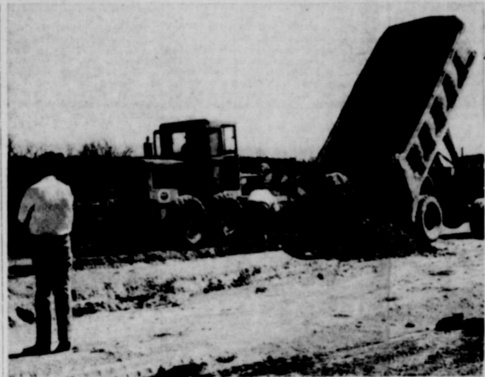
AIRPORT IMPROVEMENTS — Workmen are pictured as they place base material on the runway at the Ranger Airport in preparation for paving the north-south runway. The paving project is being sponsored by the city and the chamber of commerce. Several fund-raising campaigns are being planned by the CoC to help with the cost of the project. (Photo by Capps Studio).
