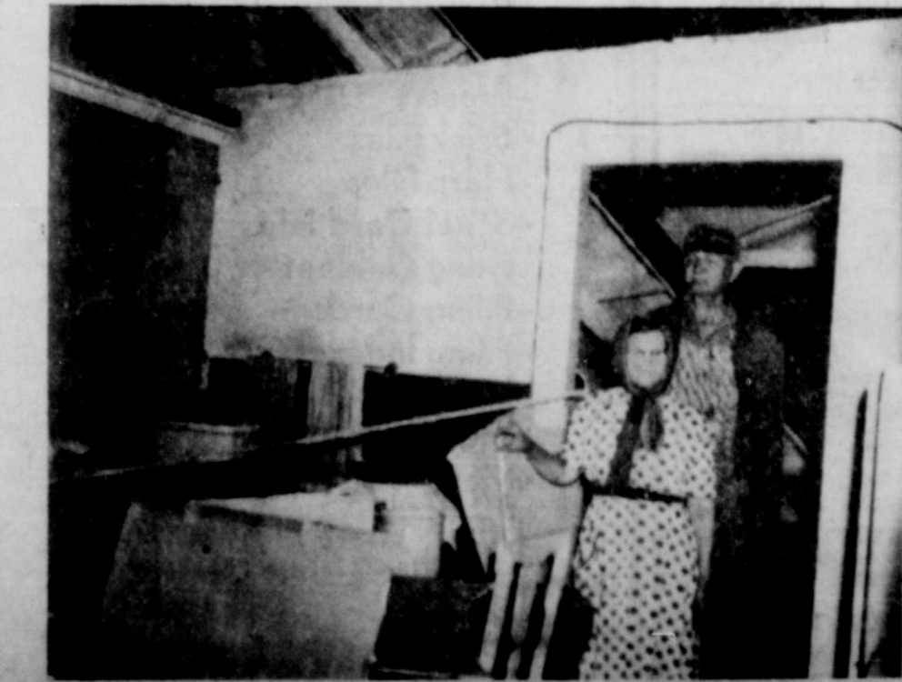
TWISTER DAMAGE to one of the rooms in their home near Eastland is surveyed by Mr. and Mrs. H. L. Gibson. The blow funneled across a corner of Eastland Lake Wednesday afternoon and snatched the roof of most of their farm residence. Mr. Gibson was slightly injured by a flying timber but Mrs. Gibson was unharmed.
