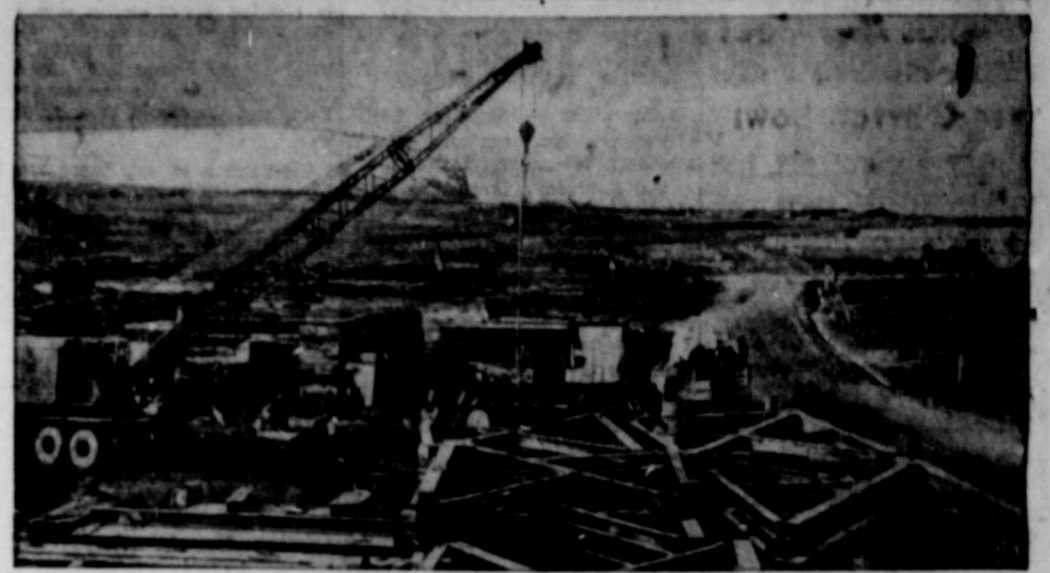
DISCLOSE AIR BASE NEAR POLE—Secrecy wraps are now off the Air Force's fantastic Arctic base at Thule, Greenland. The 90,000-acre, $263,000,000 project is only 930 miles southeast of the North Pole. Photo shows Army engineers personnel unloading steel frameworks used in construction of the base.
