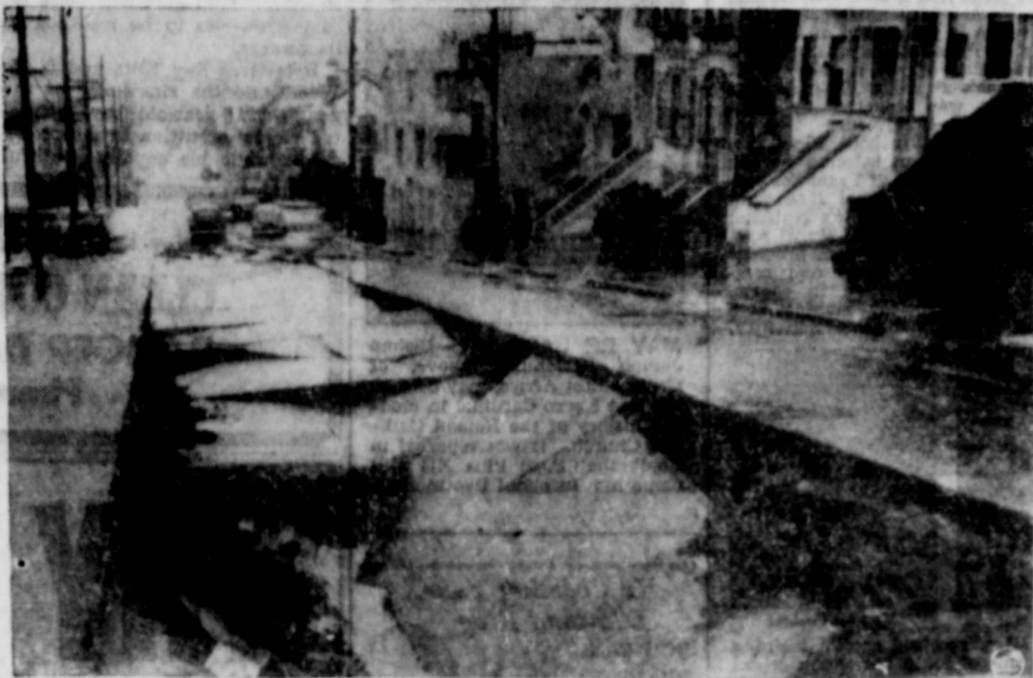
SAN FRANCISCO PLAGUED BY STORMS—This street just north-west of the downtown business area in San Francisco gave way after a heavy rainfall caused a broken sewer pipe, and the sand under the paving caved in. Already hard hit by two major rain and wind storms, the Bay area has been promised another by the weatherman. (NEA Telephoto).
