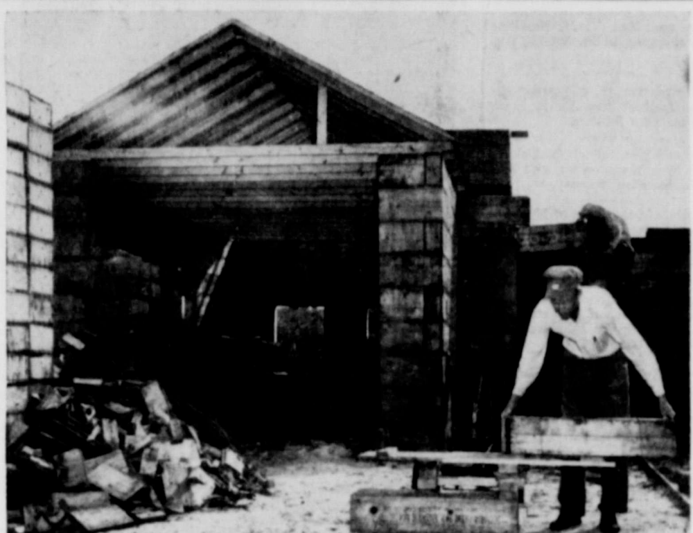
AMMUNITION-BOX ARCHITECTURE —A workman at Norfolk, Va., works on a garage he's building from Army surplus ammunition boxes. Use of the cases for building is widespread in the Norfolk area. Six hundred boxes provide enough material for a combination garage and utility room, and cost only $30.
