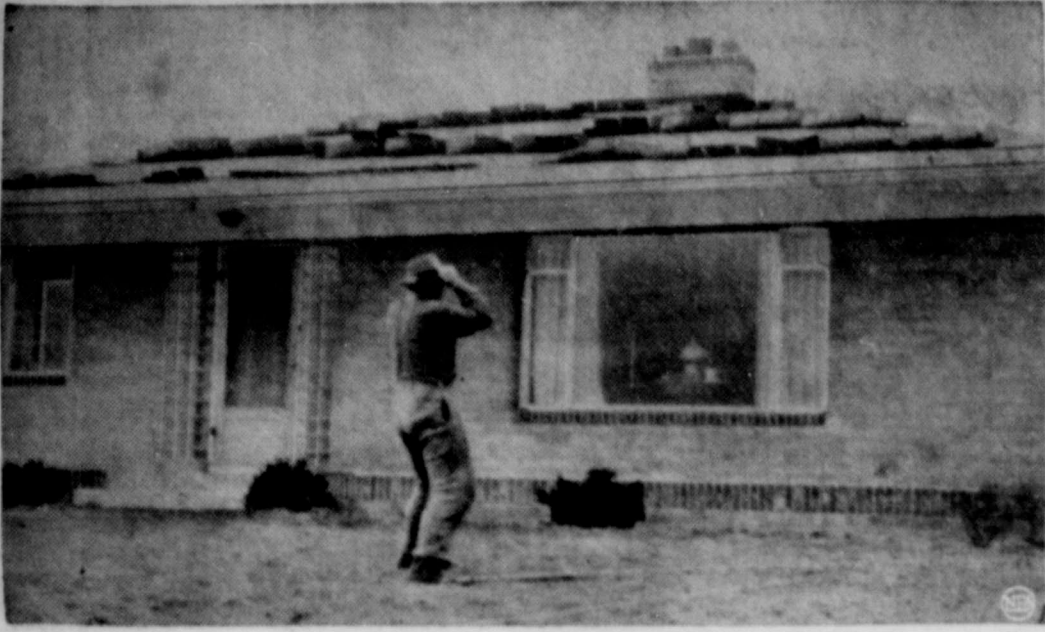
At Topeka, Kansas R. E. McConkey, crams his hat down on his head as he watches the shingles on roof of his new house stand up and prepare to take off. Winds sometimes have hit hurricane velocity in the Midwest dust storms during past few days. (NEA Telephoto).
