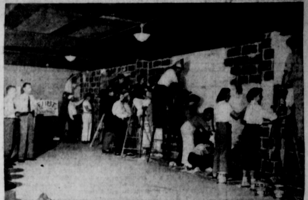
"GOOD SAMARITANS" TACKLE PAINT JOB—Almost 100 parishioners turned out at Manhasset, N. Y., to do a paint job on the interior of their new brick church. Half of the "Good Samaritans" brought their own paint brushes. The pastor, Rev. George Parker, at extreme left, directed the amateur paint artists.
