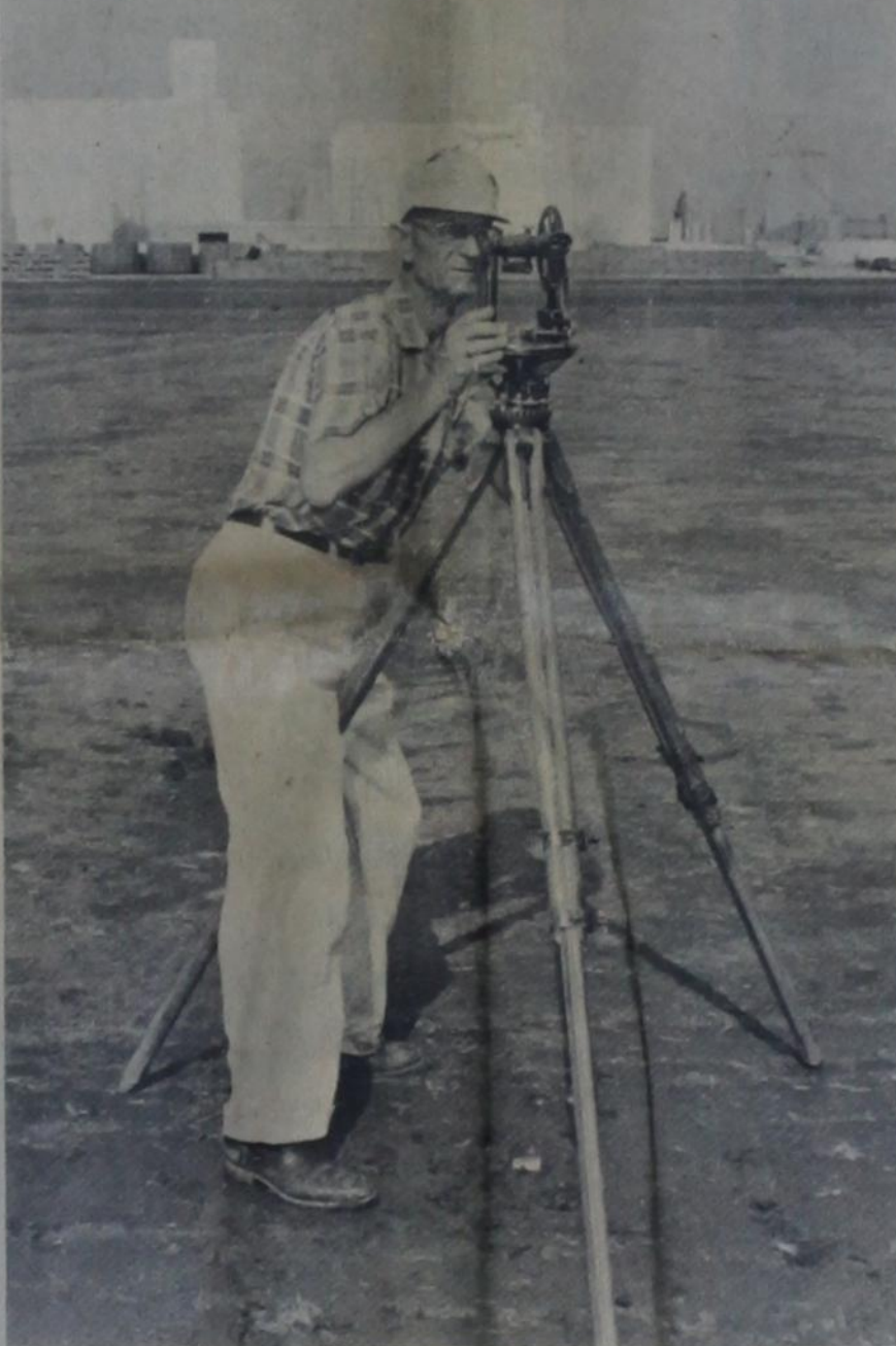
FIRST STEPS are now being taken in the construction of the million-dollar migrant labor housing project in East Dimmitt. Here, Lindsey Williams of Littlefield, surveyor for Vaughn Construction Co., focuses on the underground pipeline routes. Land leveling is now underway.
