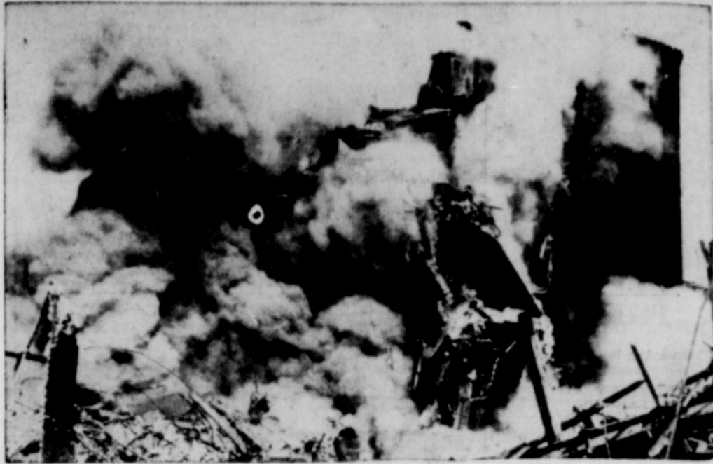
A building of the I. G. Farben plant in Ludwigshafen, Germany, damaged in the terrific blast two weeks ago, suffers further destruction — this time at the hands of the U. S. Army Engineers. Building which were dangerously near collapse were torn down to prevent additional casualties. — (U.S. Signal Corp Photo from NEA Telephoto).
