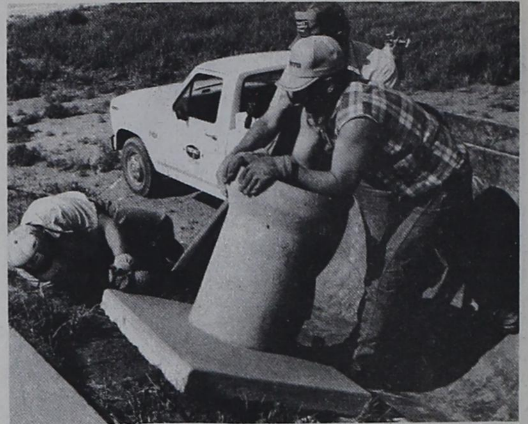
P.O.W. FOUNTAIN MOVED —Precinct 3 workers remove the 46-year-old water fountain from the end of the officers' swimming pool at the former Hereford POW Camp, in preparation for moving it to the Castro County Historical Museum, where it will be set up near an old barracks building from the camp. "We're going to try to replumb it and get it working before we set it up," Precinct 2 Commissioner Jeff Robertson said.
