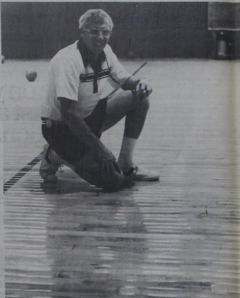
RUB-A-DUB —You could scrub your laundry on Dimmitt High School's gymnasium floor right now — and it looks as though someone already has. Coach Ken Cleveland shows the result of a recent roof leak that left virtually the entire surface of the main court in this condition. The gymnasium roof was being
