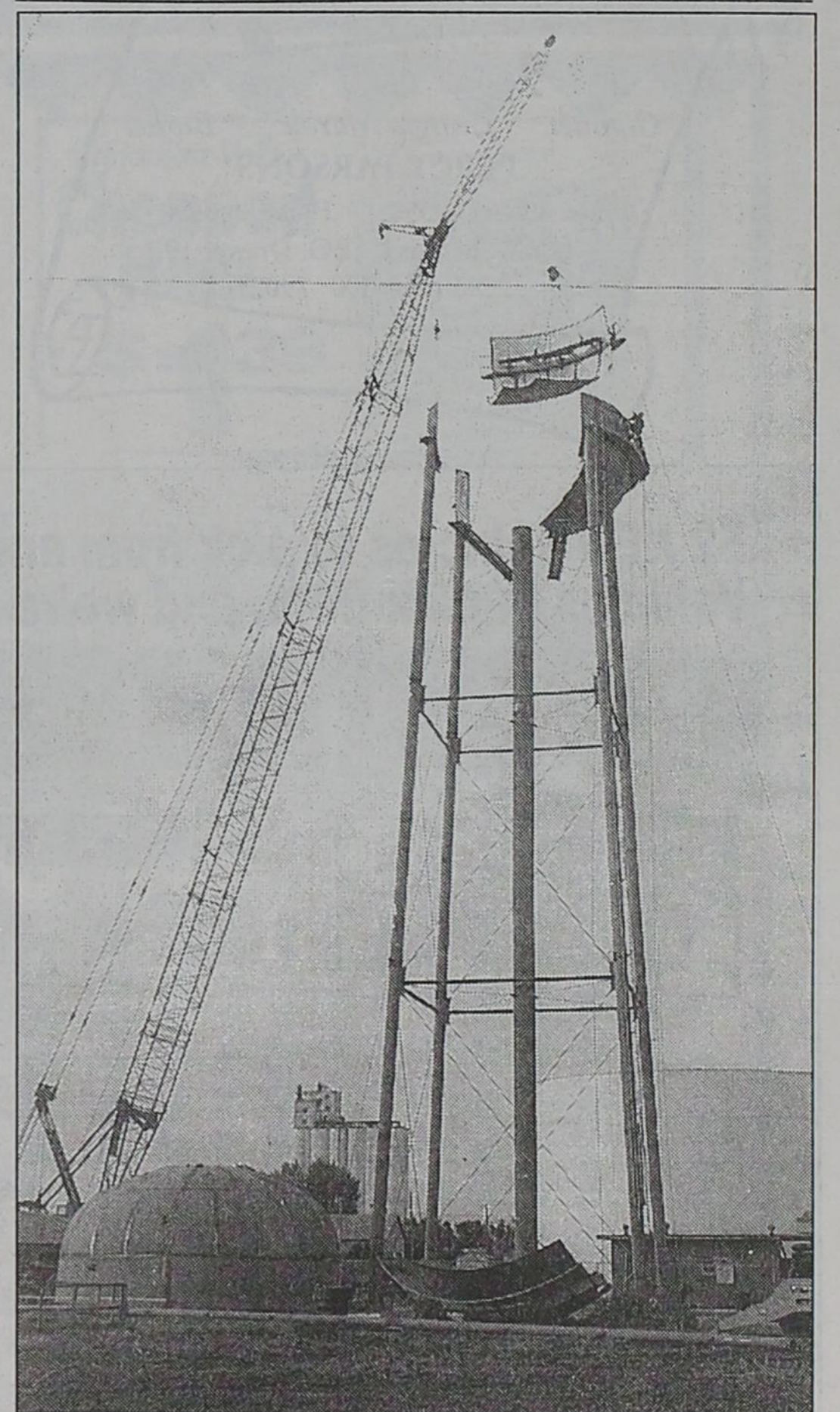
PIECE BY PIECE—The new water tower in southeast Dimmitt is being constructed by Caldwell Tanks of Louisville, Ky. The completed structure will hold 115,000 gallons. Henry Vernon, head of the work crew, said the crane will lift 14,000 pounds of steel when the "crown" is put on the tank.
