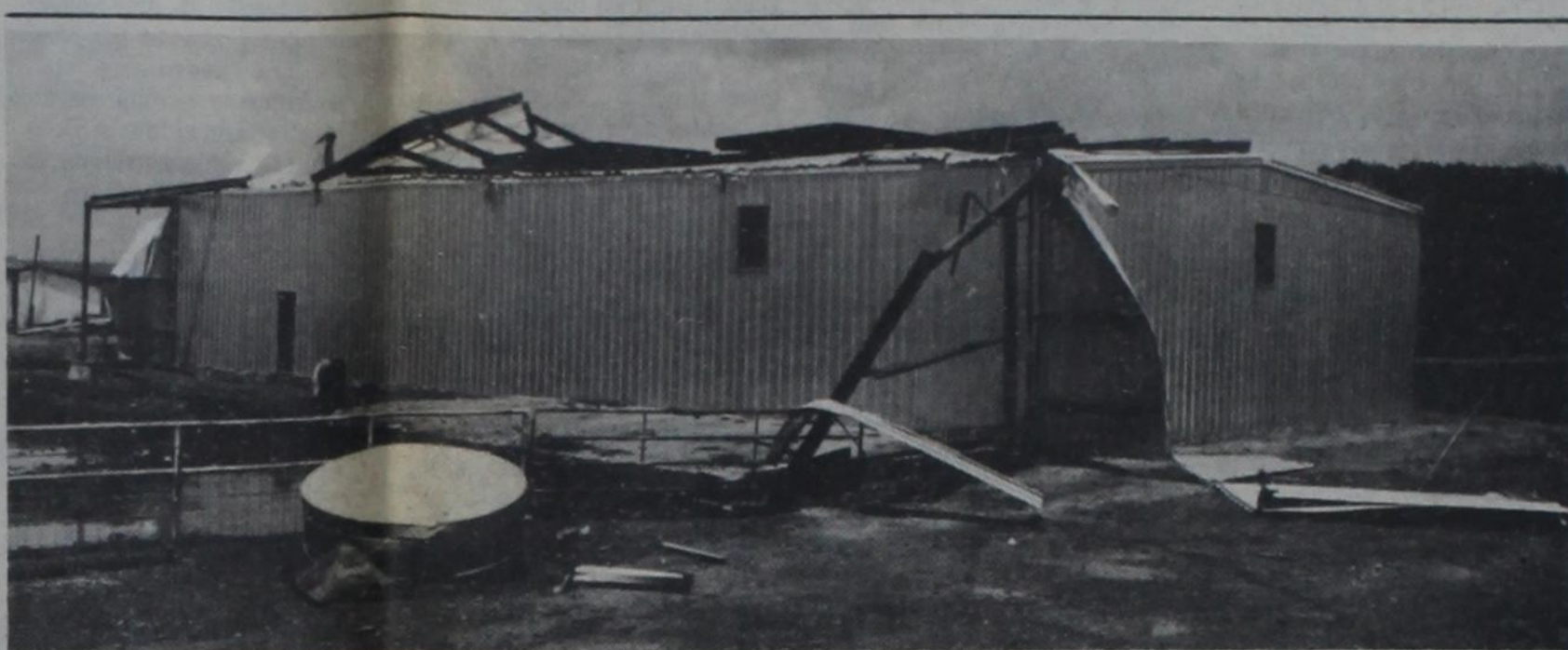
STEEL STRUCTURE UPROOTED—A mysterious high wind Friday evening uprooted the animal shelter attached to this new barn at the W. J. Martin farm four miles west of Flagg, and hurled the entire structure—steel beams and all—onto the roof of the barn, catapulting the half-ton steel pillars into a field on the other side. The industrial-grade steel barn was completed only four months ago to replace a barn that burned in the same spot in February 1977.
