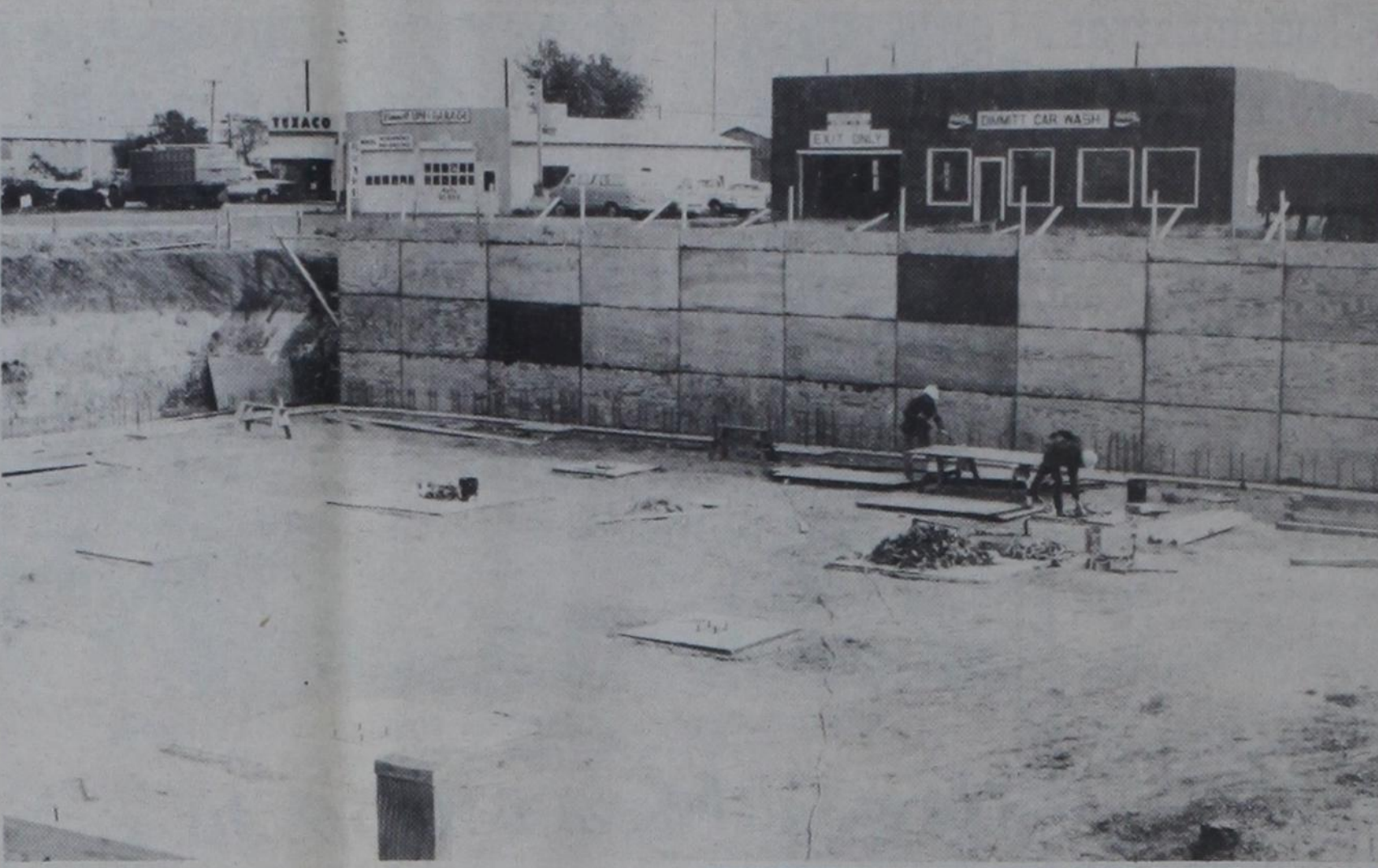
WORK IS PROGRESSING on the full-basement portion of the new First State Bank building, being constructed by the Read & Gary Strickland Co. of Amarillo. Here, workmen put up forms for the concrete walls of the basement. This portion of the building will have 9,850 sq. ft. of floor space—the same amount as the second level—and will house the bookkeeping department, storage vault, coffee room and meeting room. The bank has asked parents to warn their children not to play at the construction site because of the potential danger.
