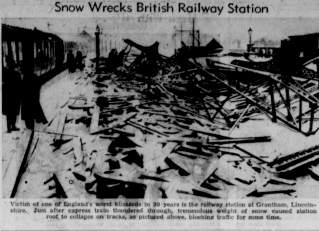
Snow Wrecks British Railway Station Victim of one of England's worst blizzards in 30 years is the railway station at Grantham, Lincolnshire. Just after express train thundered through, tremendous weight of snow caused station roof to collapse on tracks, as pictured above, blocking traffic for some time.
