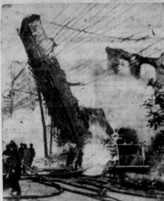
Quick action of an alert photographer got the above picture of collapsing wall in five-alarm fire at paper mill warehouse in Manayunk, Pa., where loss in salvaged waste paper alone was valued at $50,000. Seconds after photo was made, three firemen lay injured by debris from the wall.
