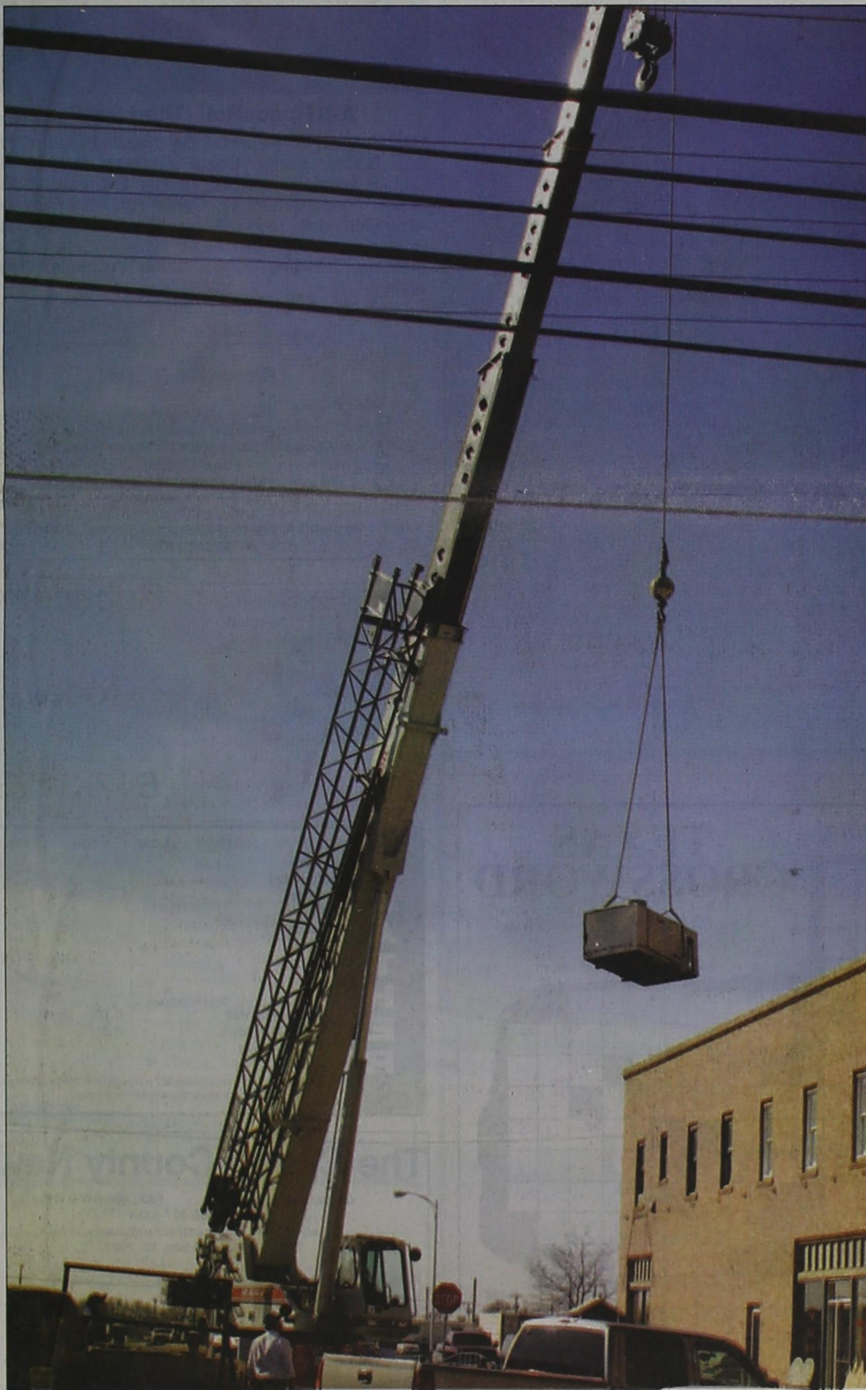
With Marvin Bryant on the ground supervising, Oscar Navarro (hidden by the roof) was able to secure this old air-conditioning unit and then Bryant had it swung away and to the ground. All told, six old units were replaced with six new ones. Bryant is the owner of Bryuant Sales and Service in Dimmitt. He said this crane is capable of lifting 150,000 pounds.
