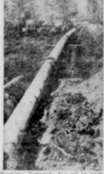
War-time demands for oil in eastern U. S. rushed construction of Plantation Pipeline to carry gasoline from Louisiana to North Carolina. Piece of pipeline is shown being lowered into three-foot trench that hides it from air attack.
