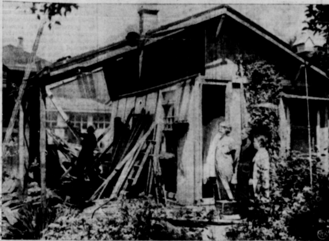
It looks like a prank of a tornado—but, actually, this home wrecking is man made. While Mrs. Minnie Behning and daughters stand by helpless, workmen tear half their North Chicago house away. Reason: part of home stood on lot lost to Home Owners Loan Corporation on foreclosure.
