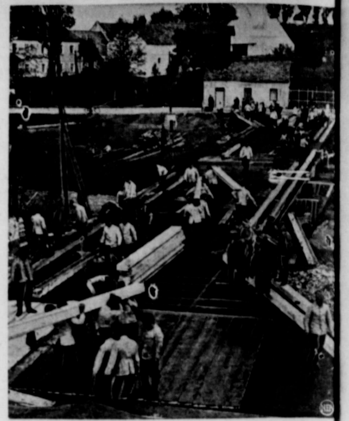
German workers in the newly acquired Sudetenland are kept busy repairing damage done during the recent crisis. Here they build a new bridge at Freiwaldau.
