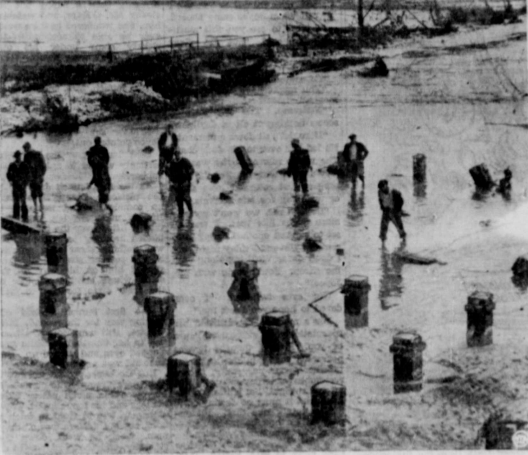
The projecting timbers seen above were all that was left of a house at Whitestone, Ga., where a cloudburst struck like a giant knife, sliced the house cleanly off its foundations, killing 13 people. This was the greatest single tragedy in the spring floods which, though dispossessing 20,000 in Alabama, Georgia and Mississippi and ruining crops in the region, took surprisingly small toll of life.
