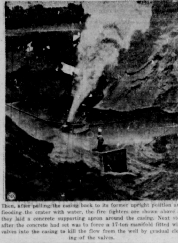
Then, after pulling the casing back to its former upright position and flooding the crater with water, the fire fighters are shown above as they laid a concrete supporting apron around the casing. Next step after the concrete had set was to force a 17-ton manifold fitted with valves into the casing to kill the flow from the well by gradual closing of the valves.
