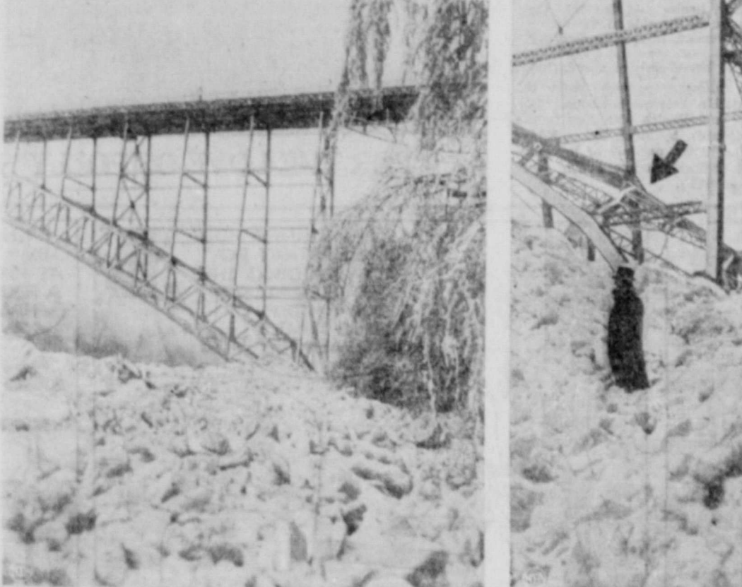
Its huge steel girders twisted and torn, its graceful arch forced out of alignment from two to three feet, historic Falls View Bridge is shown above as it resisted the tremendous pressure of the worst ice jam in Niagara's history. Pick and shovel crews battled a wall of ice 100 feet high to save the famed honeymoon bridge, for 40 years a link between United States and Canada.
