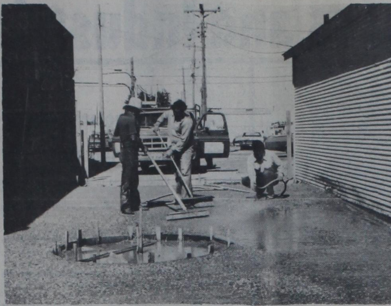
MAKING A CLEAN SWEEP OF IT —These men put the final touches on the concrete work [exposed aggregate] at the city's new mini-park Friday. The park is located in the
