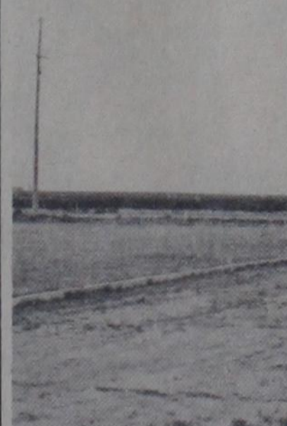
NEW STADIUM SITE—Dimmitt High School will use the same bleachers this fall, but the location and all other facilities of Bobcat Stadium will be new. Bob Campbell Movers of Hereford set the first section of bleachers into place Monday at the athletic field south of DHS. The Dimmitt School Board, which voted at its May meeting to move the stadium, is now getting bids for electrical work, ticket booths, fencing, and a new
