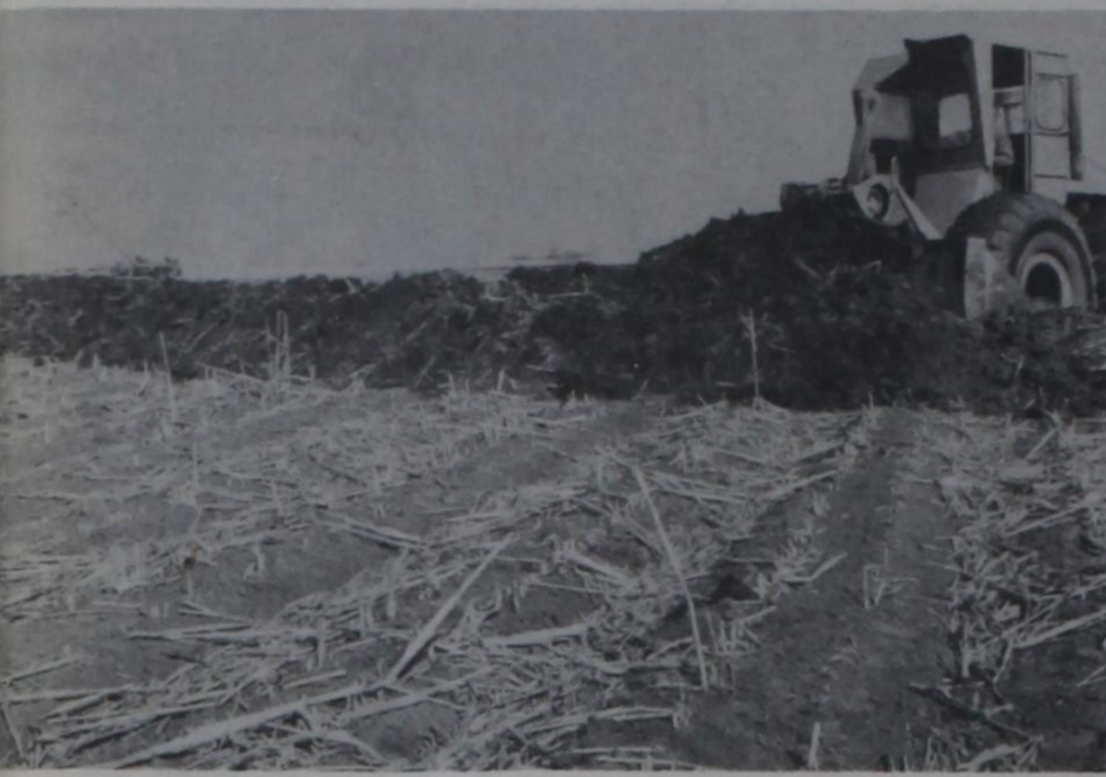
CONSTRUCTION OF Diversion dams is a sound conservation measure. Diversion break up long slopes and individualize slopes to facilitate irrigation, preventing erosion and silting.
