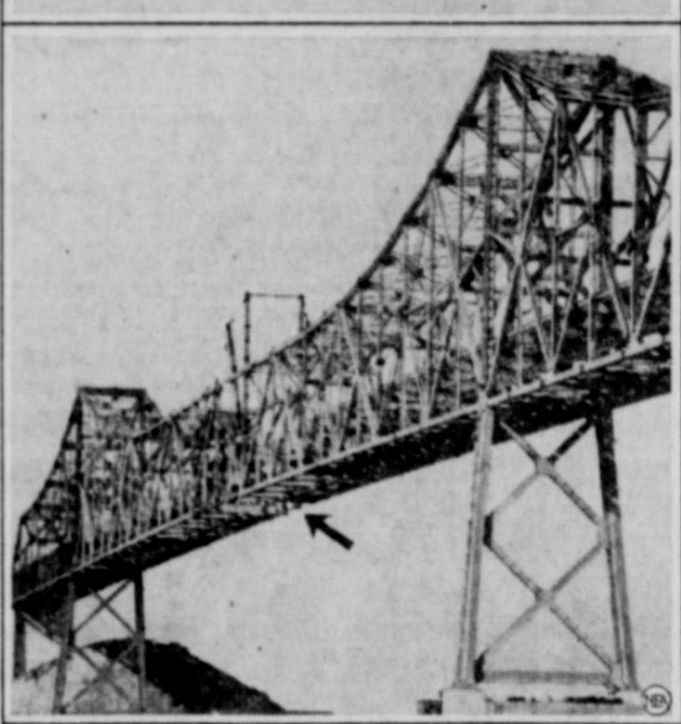
Clinging to girders and dangling from cables, workmen in the upper photo appeared like flies as they completed the difficult job of "hooking up" the last arms of the world's largest cantilever bridge, the San Francisco-Oakland Bay span. Working on their precarious perches, the bridge crews hoisted two huge eyebars simultaneously and fastened them with pins weighing several tons each. In the lower photo the bridge is shown after the last gap had been closed, the arrow pointing to the juncture. Traffic will flow east from San Francisco across the tandem-suspension bridges, through the Yerba Buena tunnel, and across this cantilever span, 155 feet above high water.
