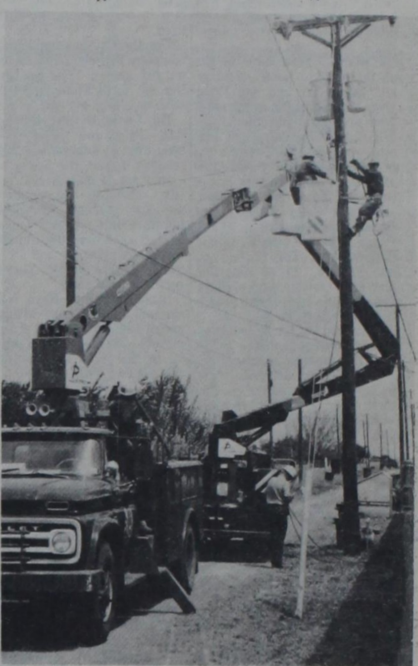
BOOSTING UP—Southwestern Public Service Co. workmen replace an old 2,400-volt transformer with a new 12,500-volt one near the Golden Spread Nursing Home during the utility's recent power conversion program for Dimmitt. Workmen, from left, are Allen Cochran, Joe Harris, Ross Mitchell, and truck driver H. W. Lowery.
