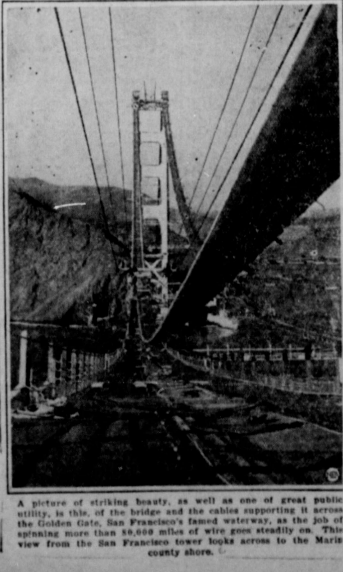
A picture of striking beauty, as well as one of great public utility, is this of the bridge and the cables supporting it across the Golden Gate, San Francisco's famed waterway, as the job of spinning more than 50,000 miles of wire goes steadily on. This view from the San Francisco tower looks across to the Marin county shore.
