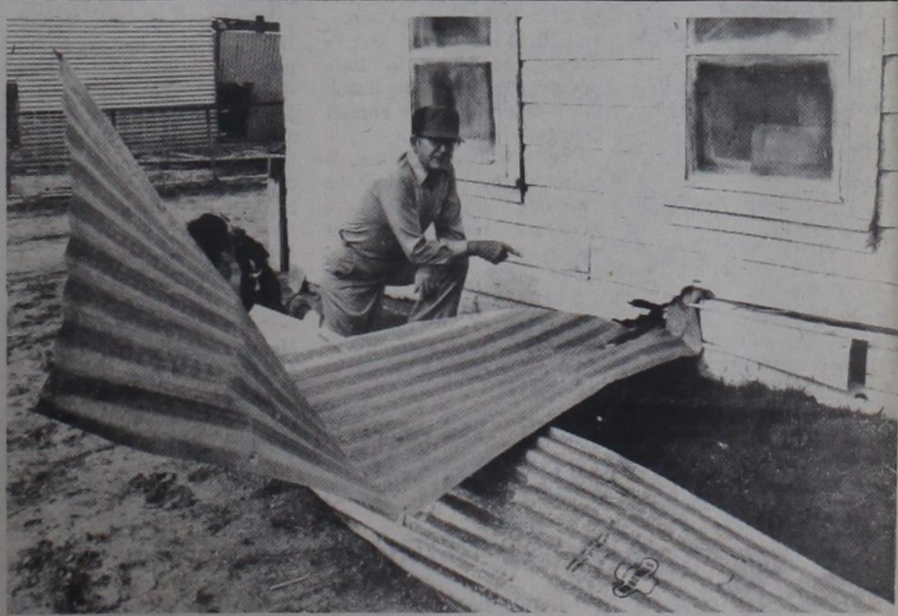
LOW AND INSIDE—Wade Mills shows where the tornado that struck his farm Monday night hurled a piece of corrugated sheet-metal through the wall of a frame cookhouse. The other end of the sheet metal is protruding through the sheetrock inside the house. The tornado scattered sheet-metal and debris more than a mile after hitting the Mills farm between Hart and Nazareth.
