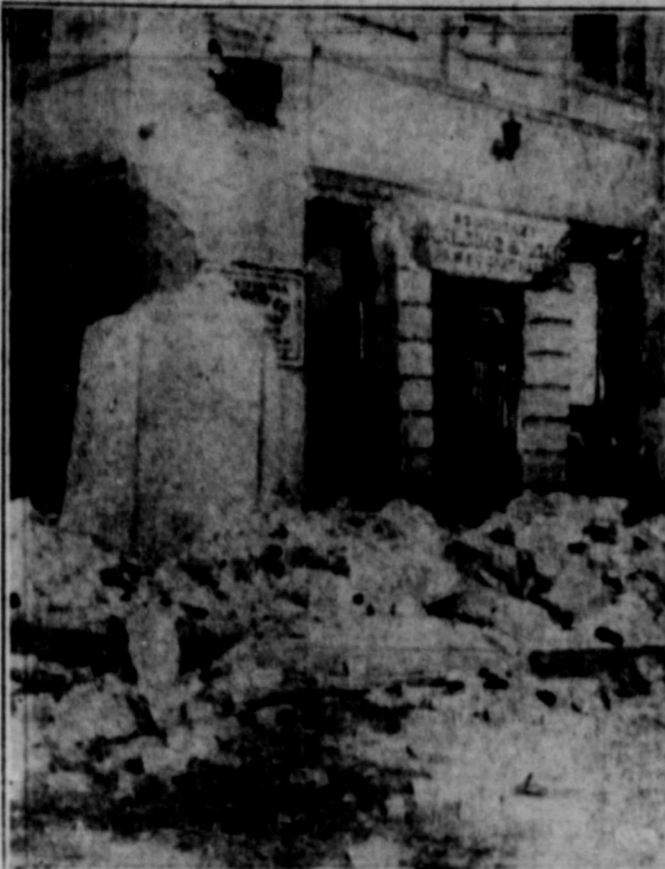
Huge blocks of stone peeling off the front of the Southwest Building and Loan Association building in Walnut Park, Calif., when it was literally shaken on its foundations by the quake.
