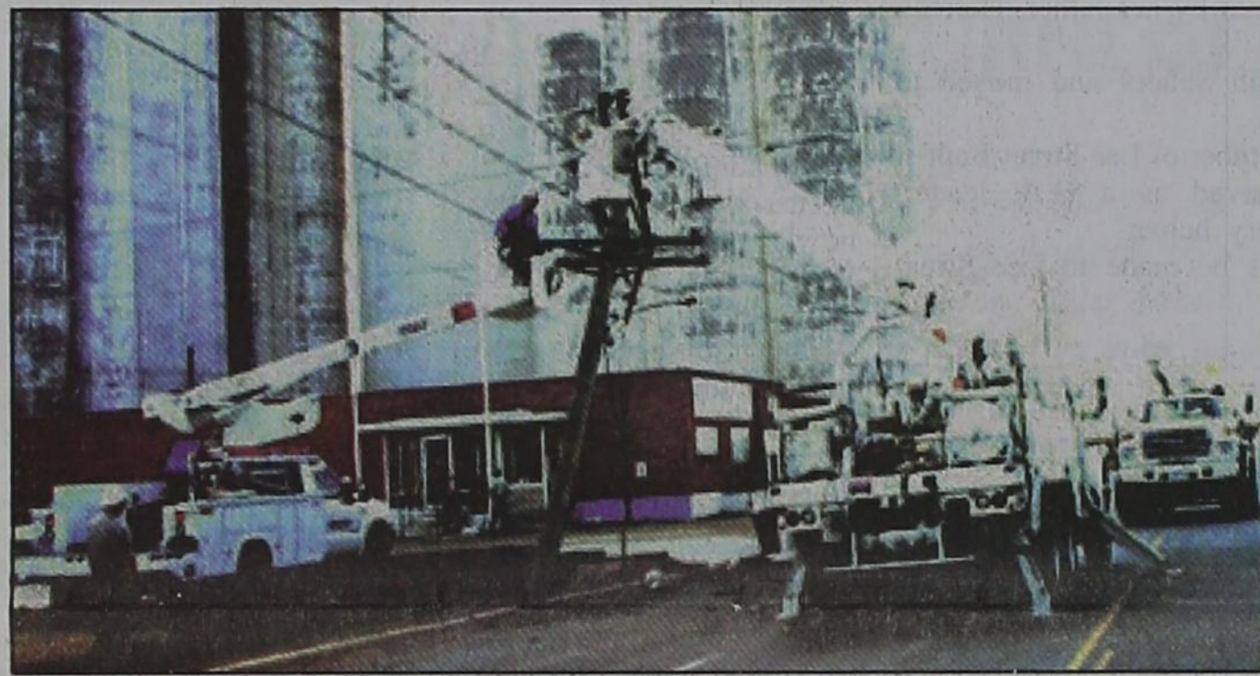
ROAD BLOCKED: Utility workers endeavor to get power back on to all of Dimmitt Monday after a late-morning accident downed a power pole. East Bedford Street was blocked most of the day.
