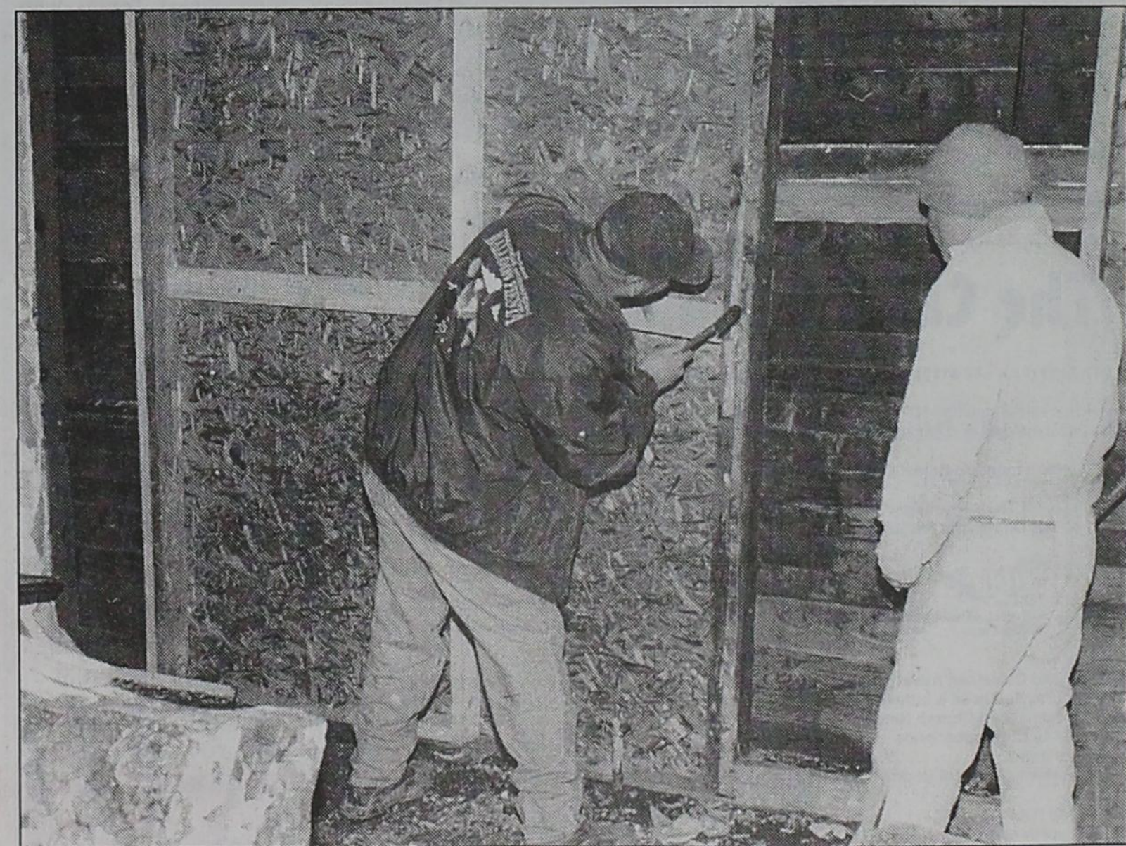
REBUILDING THE LIVING ROOM WALL —Eddie White and Ricardo Gonzales work on repairs to their residence at 207 NE Fifth in Dimmitt after it received heavy damage Saturday afternoon from what inves-
