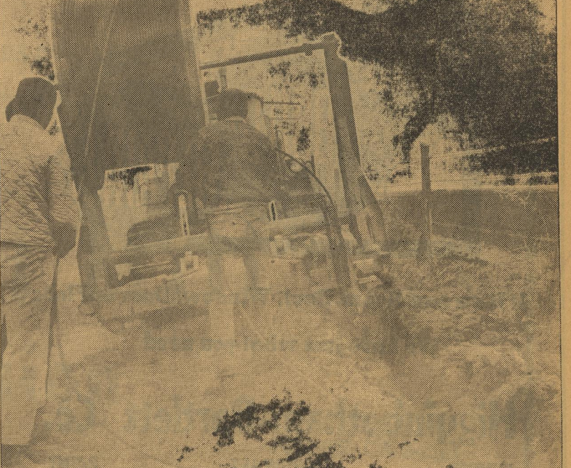
TOLL CABLE goes underground as West Texas Telephone Co. expands facilities and makes more toll circuits available. The underground cable should be completed in about 60 days according to Bill Woodard, manager of West Texas Telephone Co. See story. —Staff Photo
