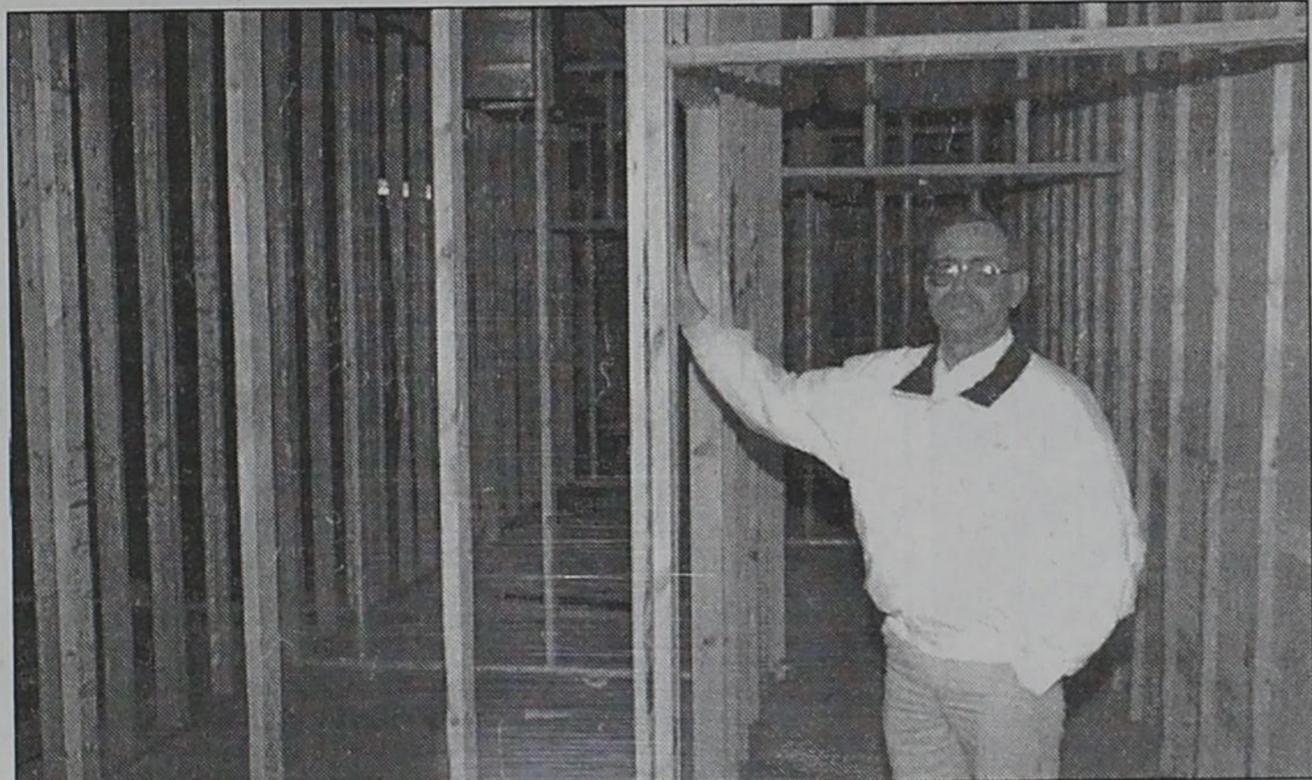
Art Benaluna checks the progress of remodeling for the hospital's durable medical equipment store which he will manage. The store will be in the east end of the Medical Center of Dimmitt building, where Edwards Laundry formerly was located.
