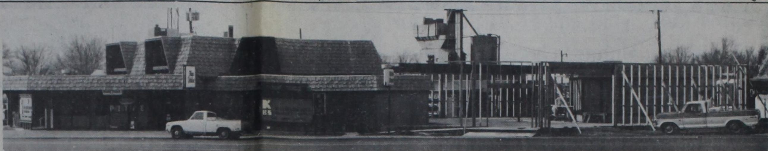
EXPANDING—Killingsworth Builders Supply in Dimmitt is adding approximately 3,300 sq. ft. more display space for its Killingsworth True Value Hardware and Radio Shack departments.
